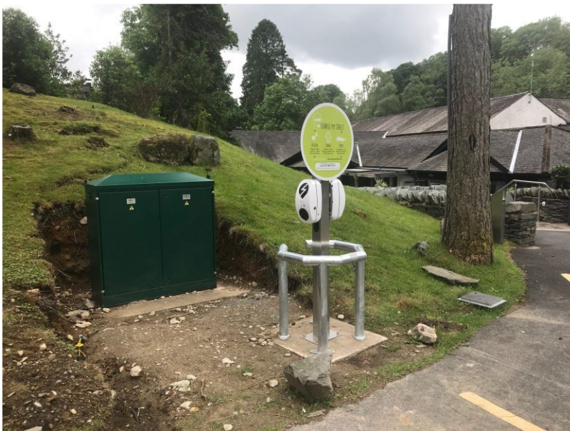
Figure 6 – Chargepoint at Langdale Leisure
