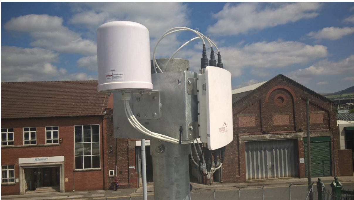
Figure 2 - lamppost with active equipment attached
